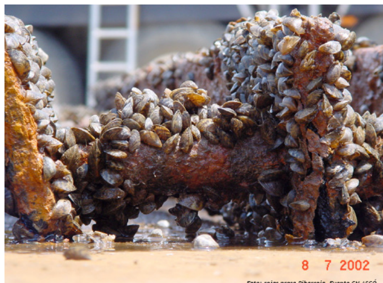
Figure 2. Metal bars from Ribarroja reservoir (Photograph by Nuclear Power Station of Ascó)
